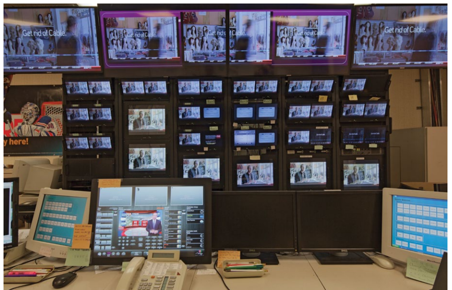
A mix of old and new control touchpanels.
