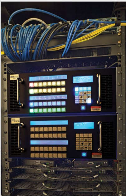
Twelve single mode fiber transmitters provide 4K signals to each of the projectors.
